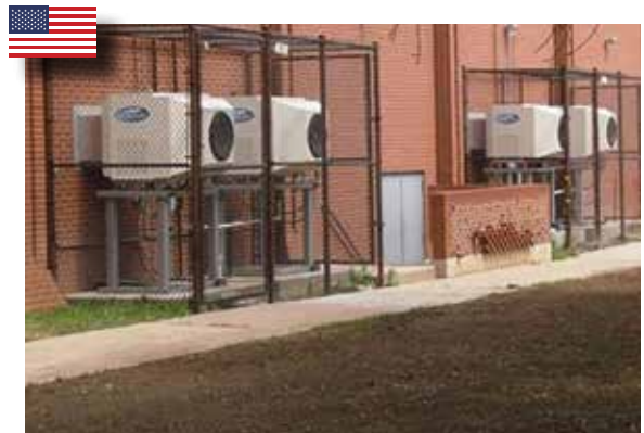
Fort Carson Army Base United States | Coolerado | Stand-alone Cooling
