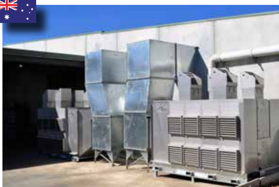
Torresan Estate Wine Storage Australia | The Climate Wizard | Stand-alone Cooling
