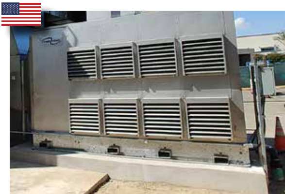
Burbank Power & Water United States | Coolerado | Stand-alone Cooling
