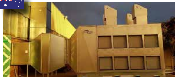
Mayne Pharmaceutical Warehouse Australia | The Climate Wizard | Stand-alone Cooling
