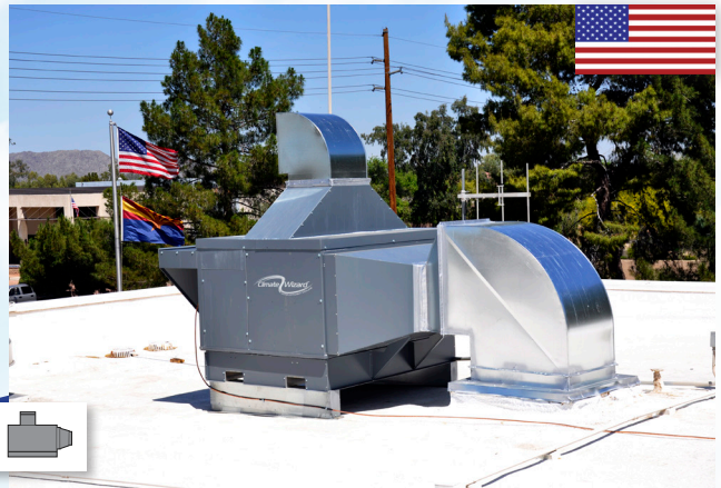
CHANDLER FIRE STATION Phoenix, Arizona, USA
